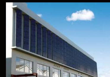
Factory facilities are equipped with our photovoltaic systems.
