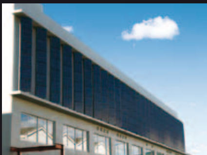
Factory facilities are equipped with our PV systems.
