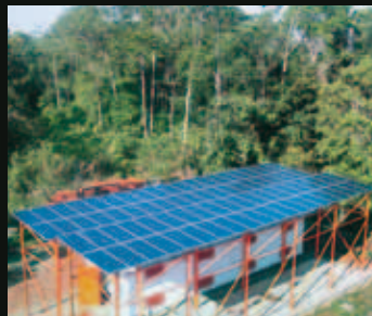
Remote telecommunications base station
